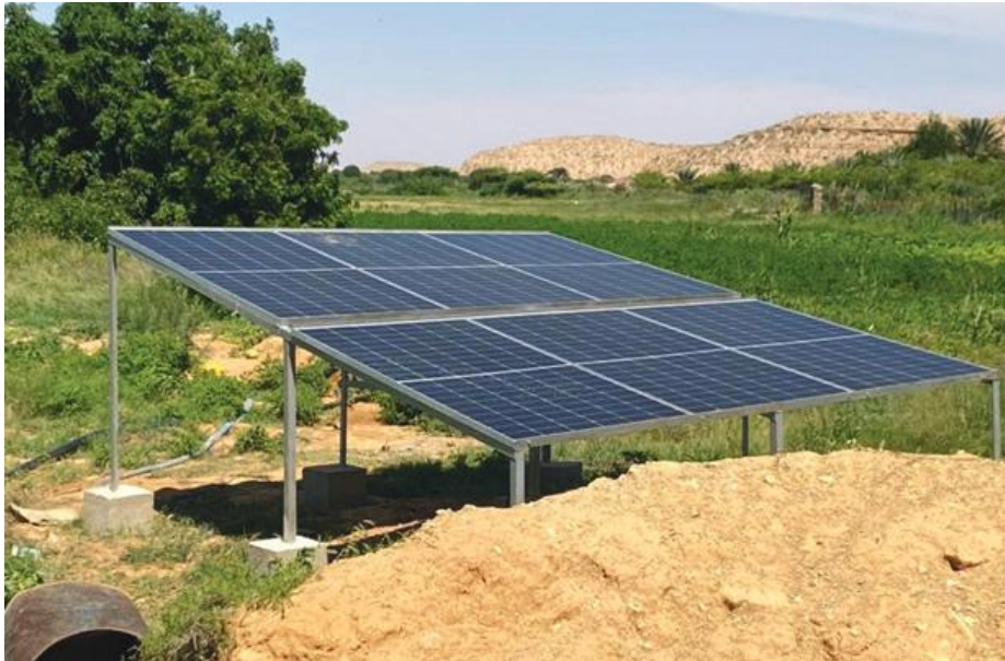
Figure 1: Completed solar system installed at Cuun site.
